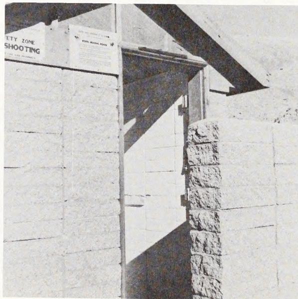
This photo shows damage to the door, shelves and Women sign. The Men's side was similarly damaged.
